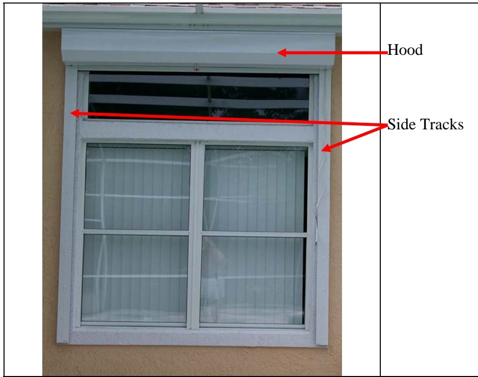
Figure G2-2 Roll shutter installed
